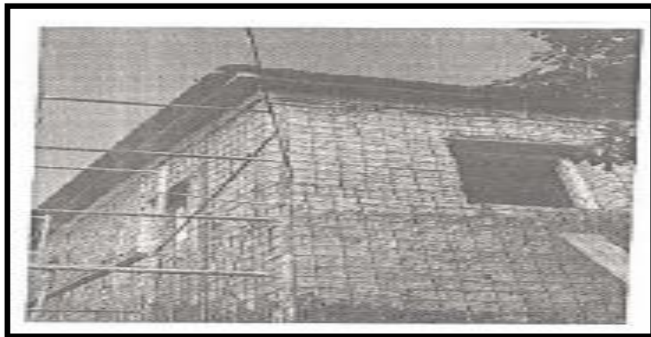
Figure 2: Reinforcement of old or damaged stone building using internal and external reinforcement coated with a layer of soft concrete (Hwajja, 2005)
